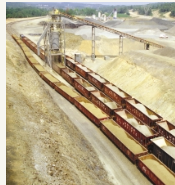
Jones Mill — Malvern, Arkansas The new automated rail loadout system can accommodate a 100-car train, delivering reduced transportation costs and greater efficiency.
